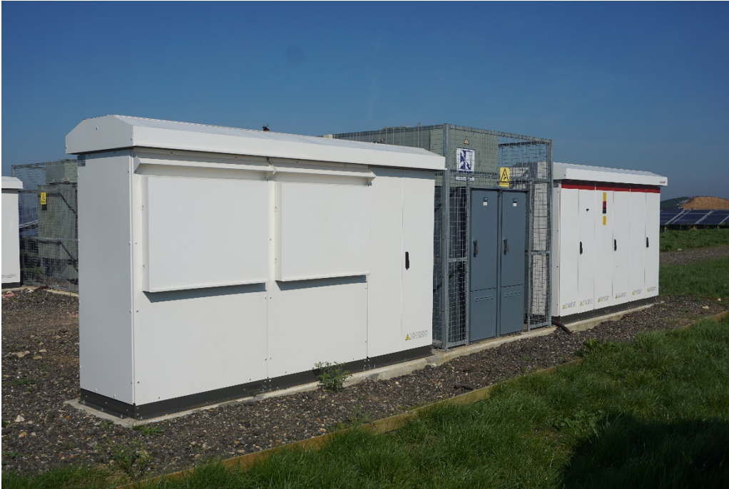
Plate 4 - Example of Solar Station located on a concrete pad surrounded by permeable hardstanding
